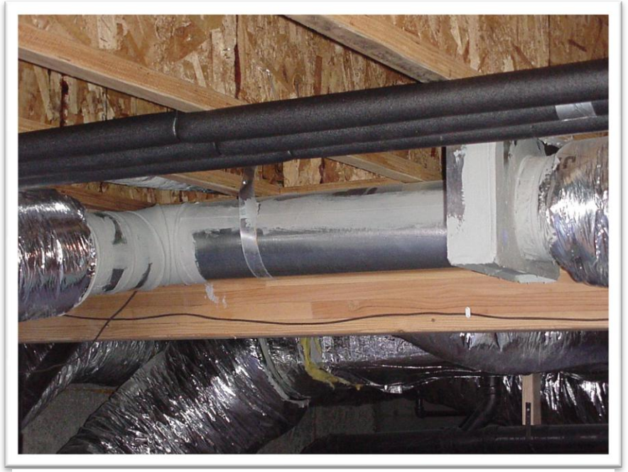
Ductwork sealed with mastic and located in a unventilated, semi-conditioned crawlspace that is part of the home's "pressure envelope"
