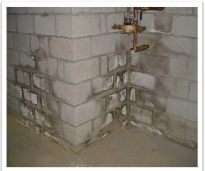
Soil moisture seeping through a stemwall damages materials and increases interior moisture levels
