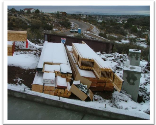
An example of how not to store building materials at the jobsite
